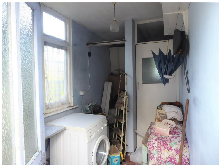
Plumbing for washing machine, w.c, sink, rear aspect window.
